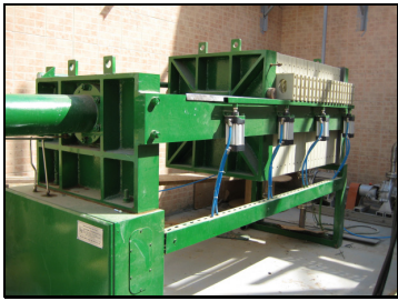
260 Liter Automatic PLC Control Filter Press Fertilizer Production Plant Abu-Rawash, Giza
