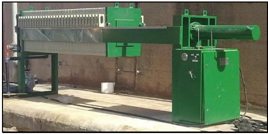
250 Liter Semi-Automatic Filter Press Sludge Dewatering, Municipal Wastewater Treatment Plant Gouna, Hurghada
