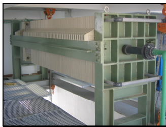
900 Liter Semi-Automatic Filter Press Hazardous Waste Treatment Plant Burg El-Arab, Alexandria
