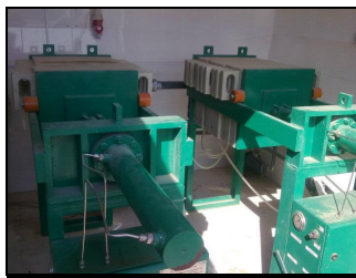
2 x 40 Liter Semi-Automatic Filter Press Waste Treatment Plant Hurghada Airport
