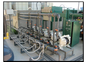
2 x 87 Liter Semi-Automatic Filter Press Industrial Waste Treatment Plant Amreya - Alexandria
